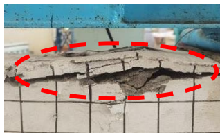
Figure 7. Concrete crushing on GM-W-200 beam
